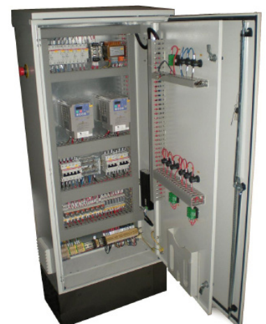
Motor Drive Unit
