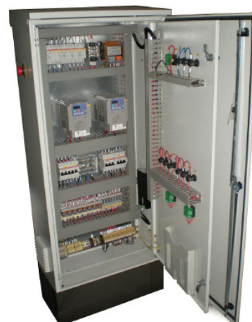
Motor Drive Unit
