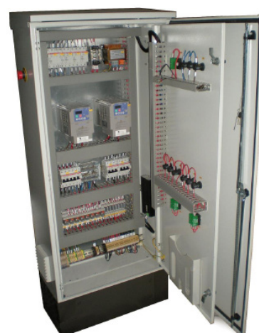
Motor Drive Unit
